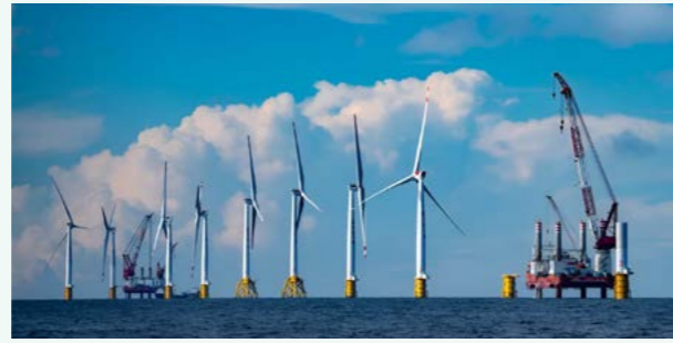
国内首个批量建设超 100 千瓦的海上风电场——阳江沙扒海上风电场 First batch construction of offshore wind farm exceeding 100 KW in China - Yangjiang Shaba Offshore Wind Farm
