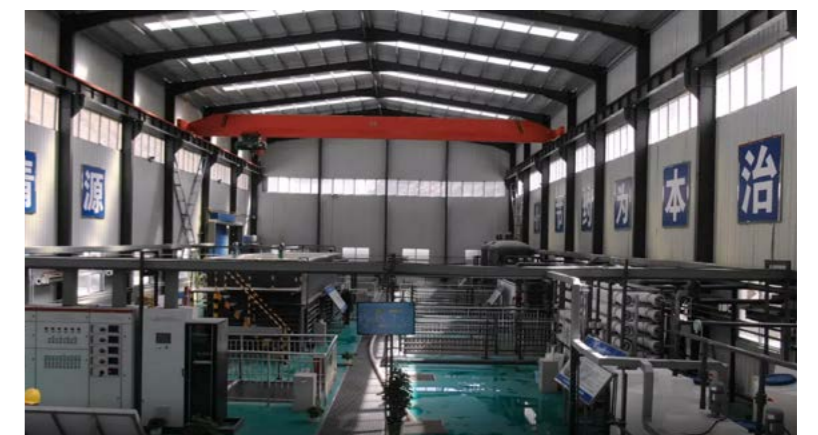
新疆天山胜利隧道生产废水处理厂 Xinjiang Tianshan Shengli Tunnel Production Wastewater Treatment Plant
